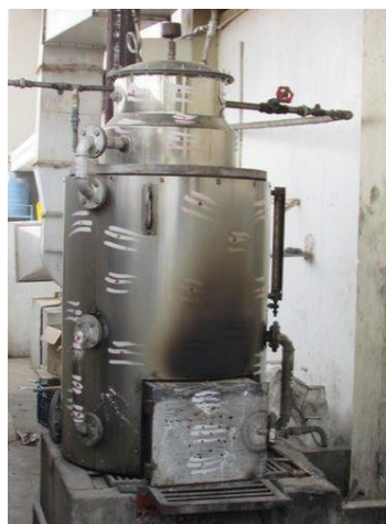
Figure: Non-IBR boiler
